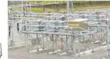
Thyristor Controlled Series Capacitor (TCSC)
