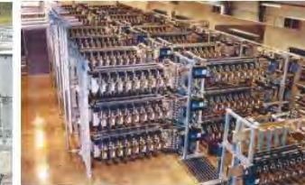
Unified Power Flow Controller (UPFC)
