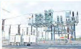
Fixed Series Capacitor (FSC)
