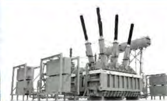
Phase Shifting Transformer (PST)
